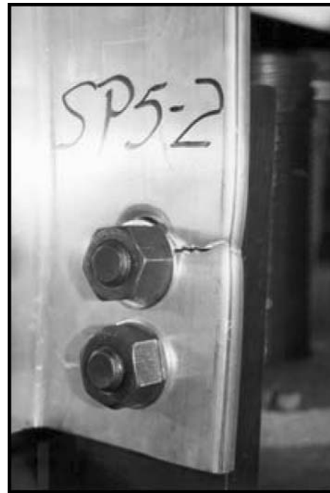
Fig. 4 Failure of a 150 × 150 × 12.5 mm angle
